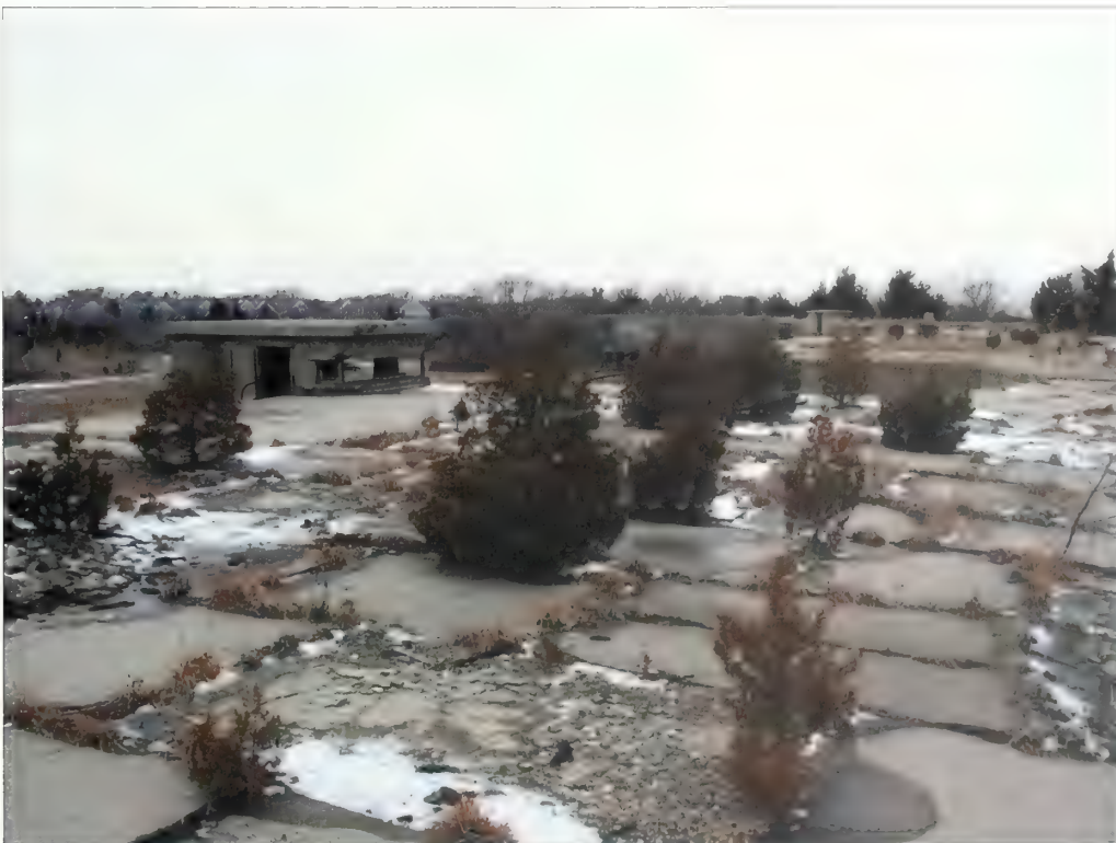
Figure 5.44. View looking west toward battery commander's station Bloomfield, Nine Gun Battery. Eastern red cedars ( Juniperus virginiana ) have become established in the joints of the concrete terreplein and should be removed (Olmsted Center, January 2009).
